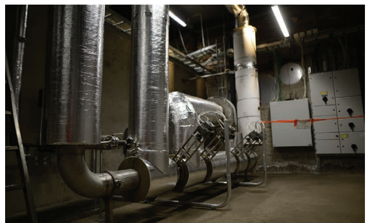
FIGURE 7 Part of the heat transfer system installed by Polar Night Energy in Tampere, Finland. The vertical pipes at left are part of the heat exchanger, while the resistive heater elements are wrapped in white insulation at right. Between these components is the air-circulating radial blower.
