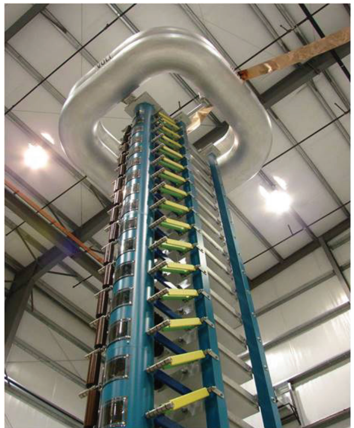
FIGURE 1 High-voltage generator (2.4 MV Marx generator) operated by NTS.
