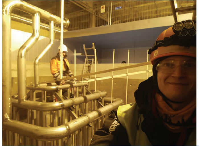
FIGURE 4 Tommi Eronen (foreground) and Ylönen inspecting the ductwork of a Polar Night Energy heat storage vessel.
